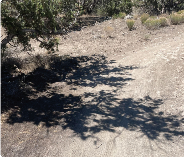
ObjID 15, Bugs Bunny: Outspread on the uphill side of Switch back heading down Hill. Berm is peeling away.
